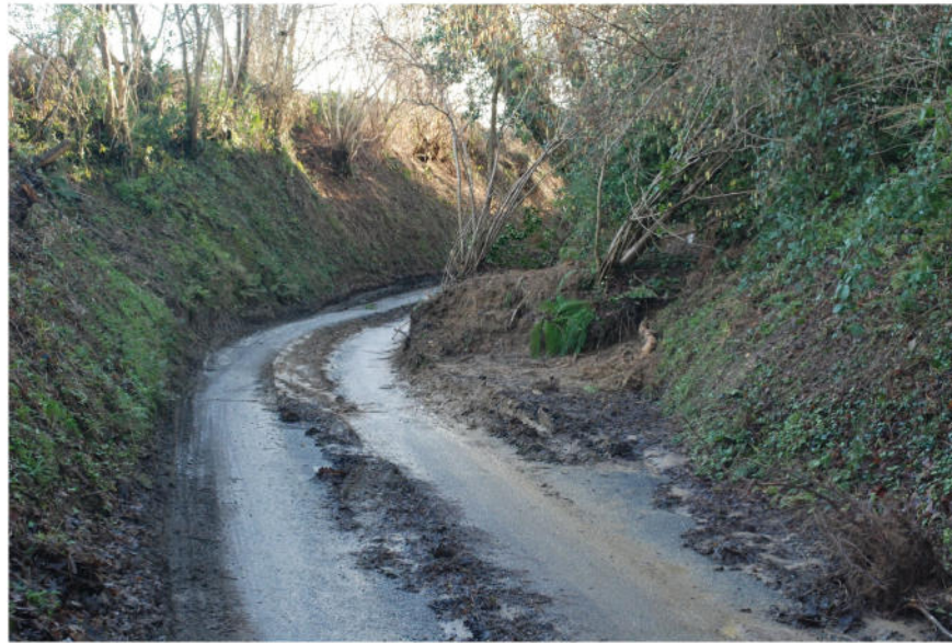
Fig. 7. Landslip in sunken lane, Stedham, West Sussex.
