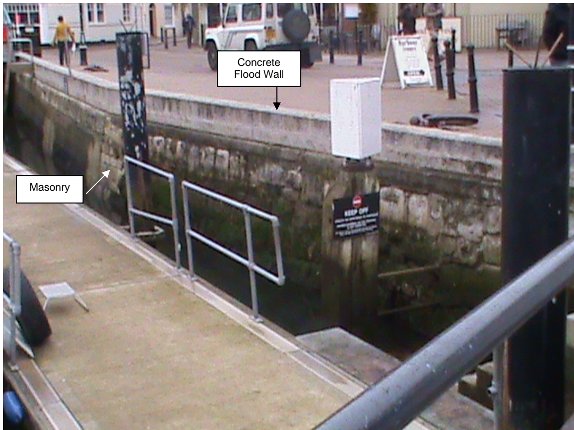
Photo 3.1 – Example of the concrete flood wall on top of a masonry wall
