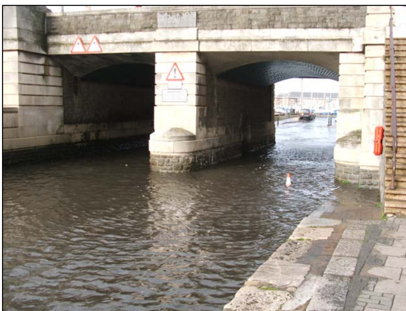
Photo 6.1 – Flooding of road beneath Town Bridge
