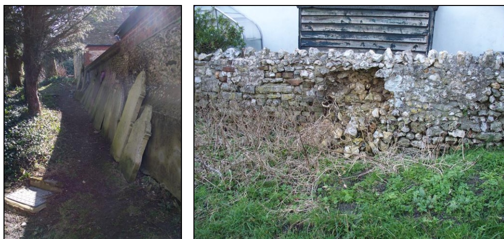
FIG. 17: Damage and decay. Left: toppled or removed headstones propped against the churchyard wall. A number of these are of eighteenth century date. Right: Collapsing flint boundary wall adjacent to No. 1 The Orchard.
