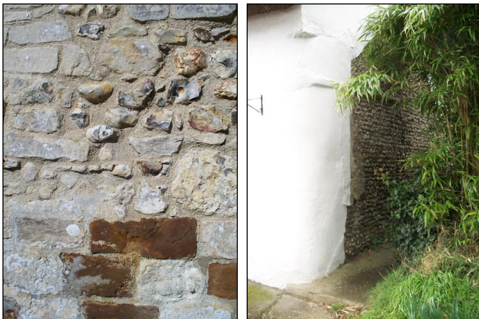
FIG. 12: Building stone. Left: a mixture of heathstone, limestone and flint used in the thirteenth century chancel of St. Christopher's. Right: Exposed gable wall of the Malthouse, which shows regularly coursed flint, though the frontage is rendered.
