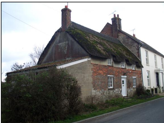
FIG. 13: Little Rhylcombe Farmhouse. The facade contains a mix of materials, showing evidence of a complex evolution: stone plinth of limestone and heathstone, with brick walls of two phases raised in cob, topped by a thatched roof. Though unsympathetic in design and construction, the concrete block extension with double roman tiled roof further adds to the mix.
