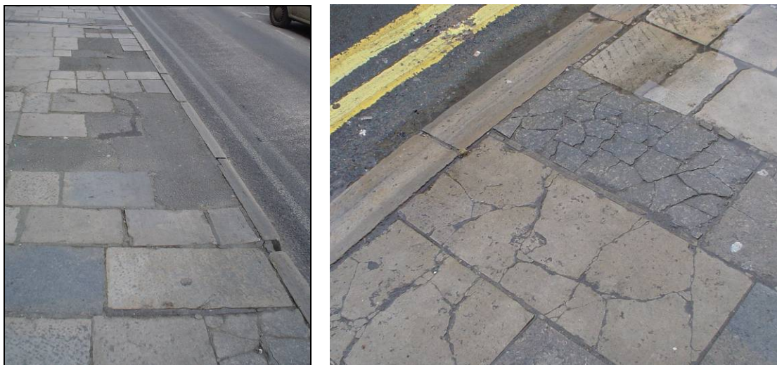
FIG. 45: Pavement Maintenance. Right: Patching of pavements using asphalt. Left: Cracked slabs where vehicles have overridden the kerb.
