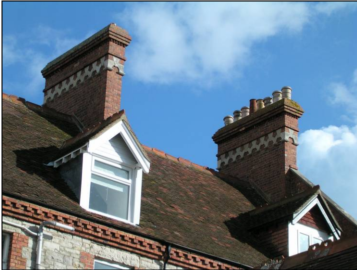
FIG. 35: Ornamentation on stacks along Cluny Crescent. Note brick cornice and dental course, also brick dressings to the windows. Dormer on the right has hanging tiles which have been lost from that to the left.
