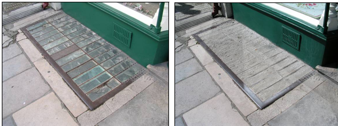
FIG. 43: Before and After. One of two pavement lights outside 50 High Street smothered with cement. These features of interest could have been repaired.
