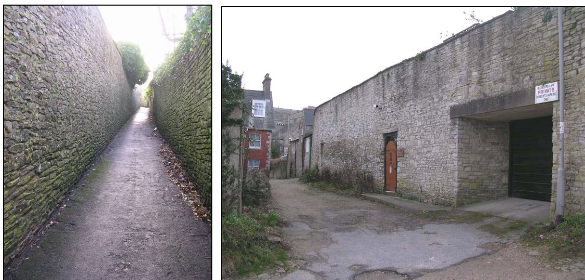
FIG. 3: Swanage walls. Left: tunnel-like quality of Chapel Lane. Right: back walls along Bloucher's Lane. Here as elsewhere the fabric has damaged in enabling infill of the gardens behind High Street properties.
