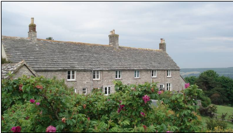
FIG. 4: 1-3 the Lane. This row of two storey cottages displays many typical characteristics. Rectangular in plan form the long and unbroken roof is here a notable feature.
