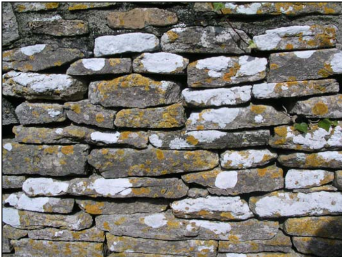
FIG. 5: Traditional walling. Fine slabs of rubble neatly coursed. Note the attractive role played by lichen, indicative of good air quality.
