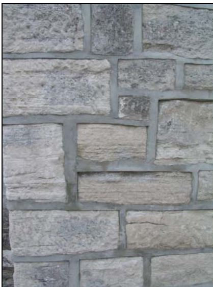
FIG. 17: Inappropriate repointing. This building has been 'pointed' using a grey cement based mortar carrying a raised 'strap' finish. It is likely that the joints have not been properly raked out and that this has been applied over the top of an existing jointing. Not only is this visually unattractive but the hard and impervious nature of the mortar will cause severe erosion of the building stone along its edges.
