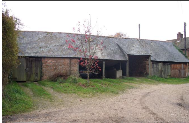
FIG. 12: Cart sheds to the rear of the barn. Buildings such as these are particularly attractive to swallows.
