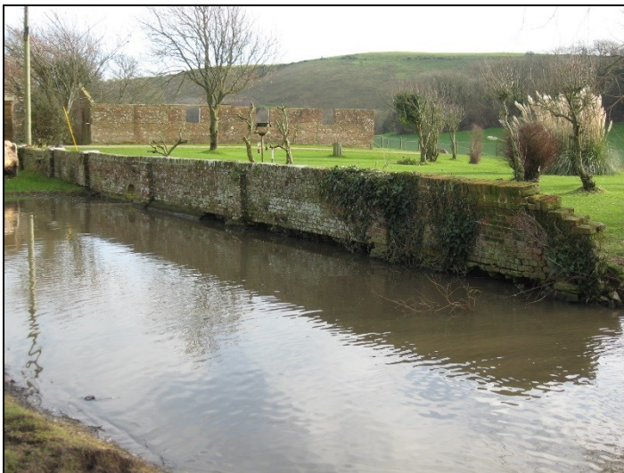
FIG. 17: Garden wall opposite East Creech Farm. The brickwork is in poor condition, being damaged by ivy and leaning in places.
