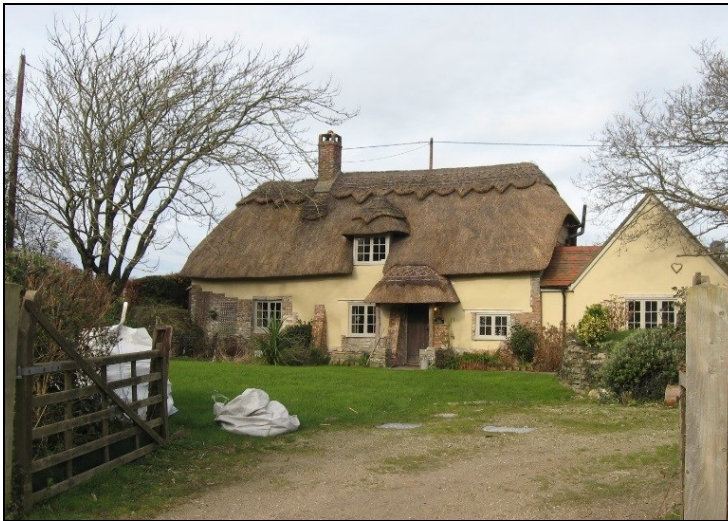
FIG. 10: Wren Cottage. The original part of the structure stands at the centre. The elaborate block ridge is not a traditional feature.
